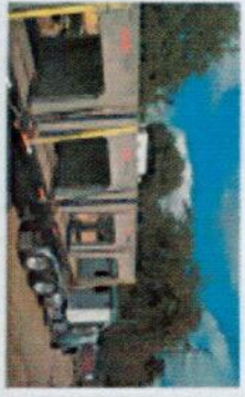
Workers install the final formwork for the stormwater BMP. The BMP will store stormwater and filter out pollutants before it enters the city's stormwater system.
